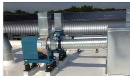
BCV Building Exhaust
